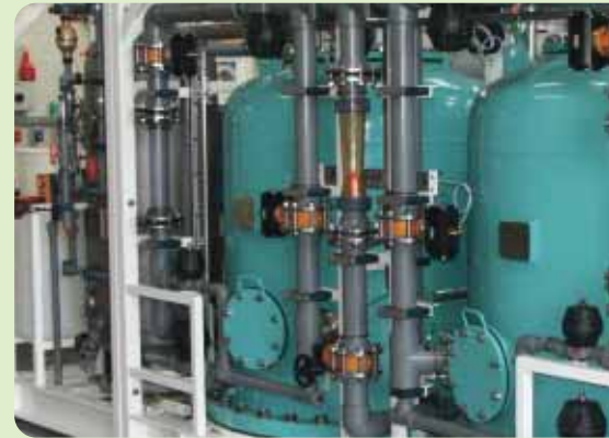
100 m 3 /day reverse osmosis desalination plant as fitted to the UK Royal Navy's Aircraft carrier HMS Illustrious.
